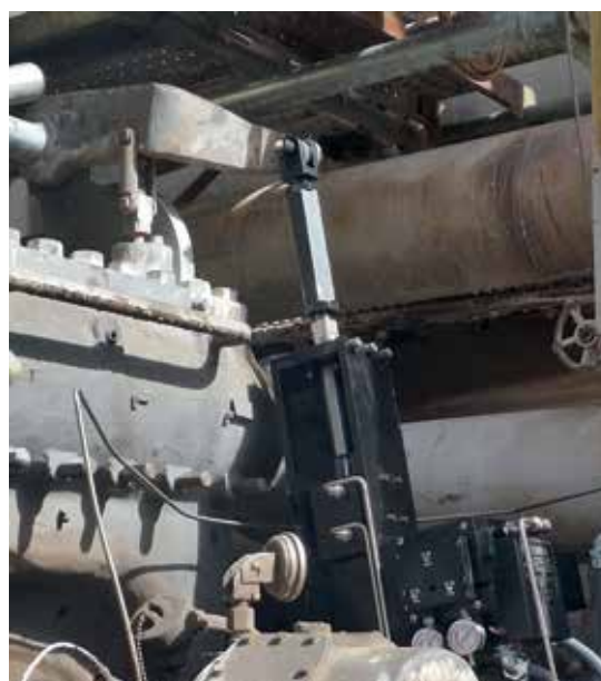
An actuator in a turbine governor application
