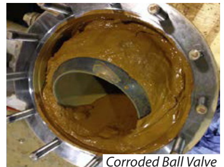
Corroded Ball Valve
