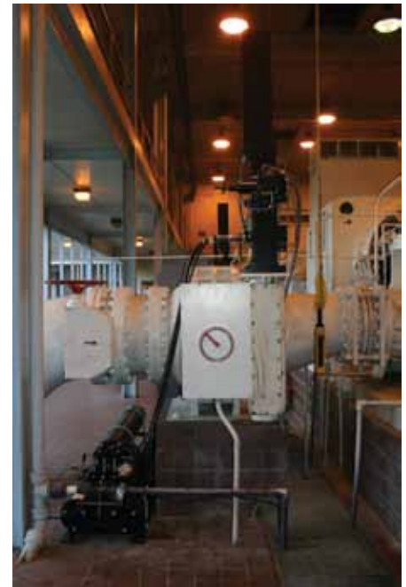
Rexa electrohydraulic (Electraulic) actuators from Koso America were installed at the City of Cocoa starting with a trial installation in 2005.
