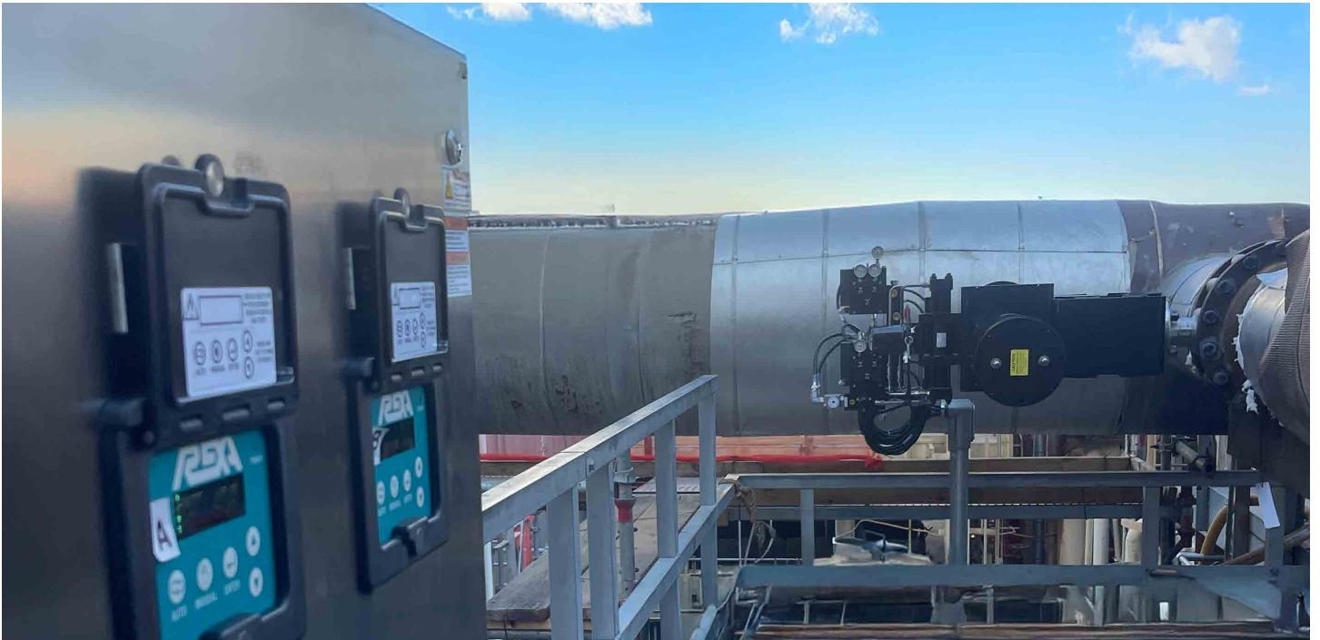
Compressor Anti-Surge Valve Control
